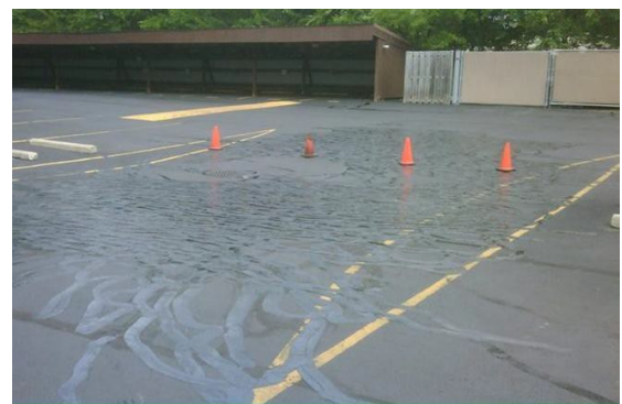
Example: Over-Applied Sealant
